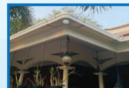
OCEAN RAINWATER HARVESTER INSTALLED
